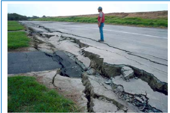
Figure 2. Lateral spreads caused by liquefaction of the soil (Photo: USGS Multimedia Gallery).
